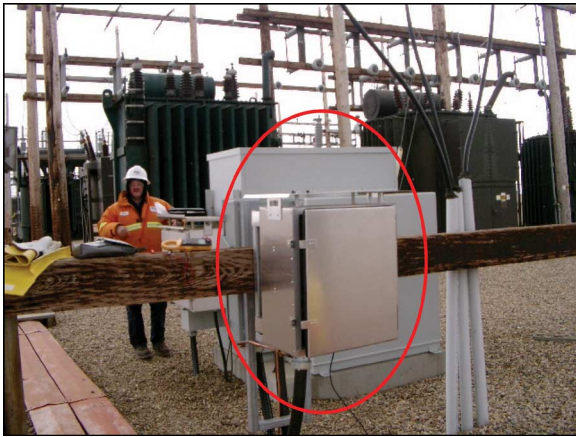
Fig. 2. Signal generator installed at the substation.
